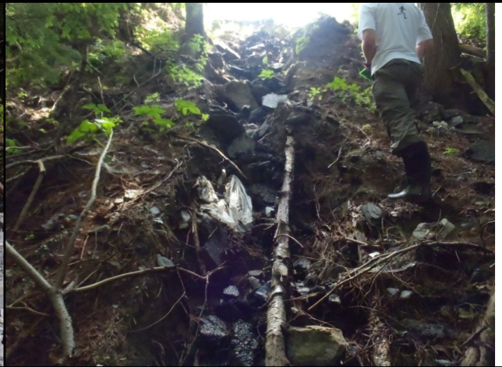
Photo 6. Stormwater flow down hillside to west, with visible erosion
