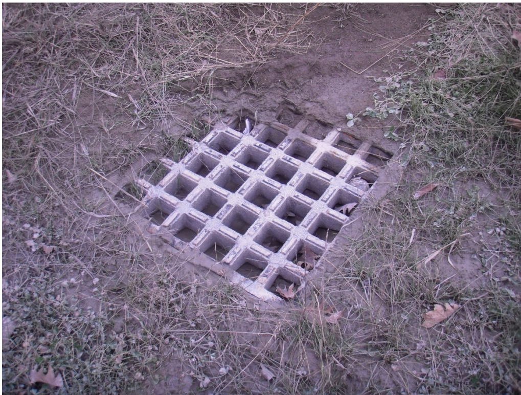
Figure 12. Sediment has completely filled catch basin at the Highgate town sand shed.
