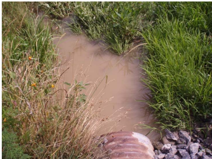
Figure 21. Scour pool at outfall from undersized culvert that carries unnamed Rock River tributary under farm road. Some rip rap has been placed by the landowner to address localized erosion around the culvert.
