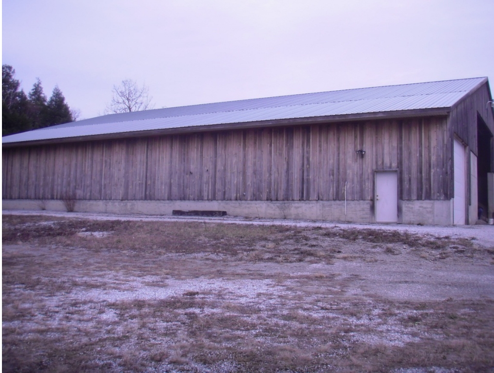
Figure 11. Town sand shed and adjacent gravel lot includes more than 0.5 acres of potentially treatable impervious surface.
