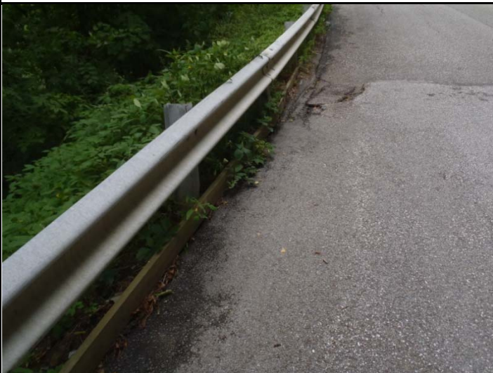
Photo 1. Erosion along roadside
