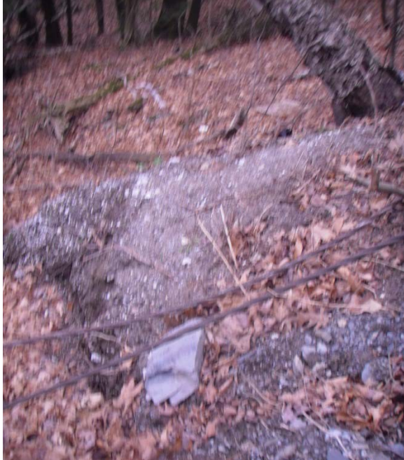
Figure 16. Erosion at the Mill Hill Rd. storm sewer outfall.
