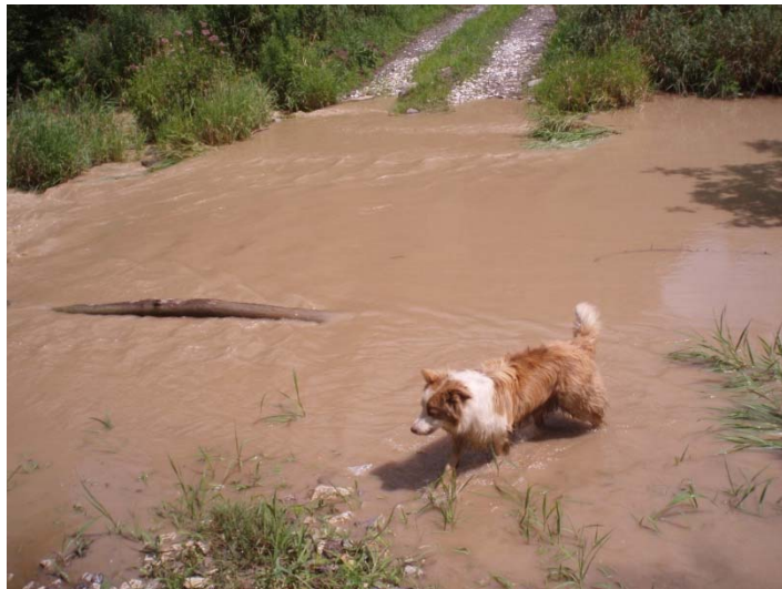
Figure 25. Unimproved farm road crossing, shown during high flow conditions. Bank erosion evident on both sides of the stream.
