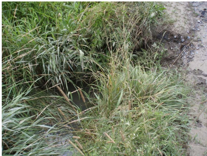
Figure 23. Undersized culvert under farm road. Erosion occurring from road surface as well as in scour pools at the upstream (shown) and downstream ends of the culvert.
