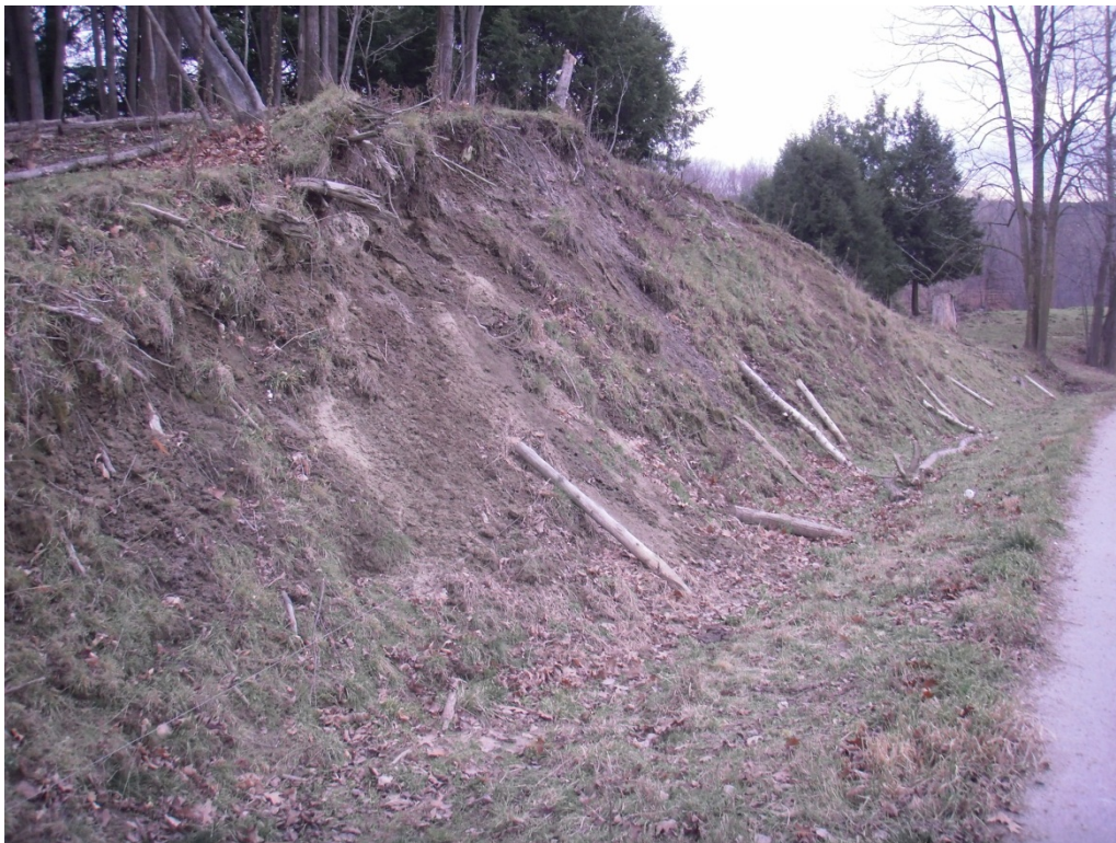
Figure 3. Eroding ditch backslope on the east side of Durkee Road in Highgate Center.
