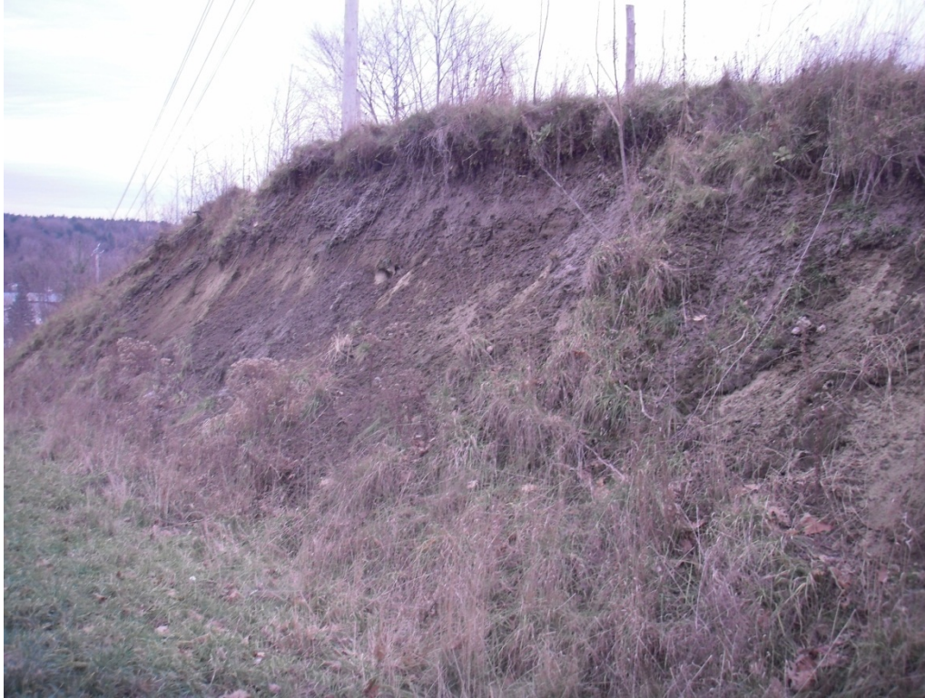
Figure 2. Oversteepened and eroding ditch backslope on west side of Durkee Rd. in Highgate Center.
