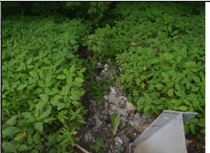
Photo 2. Blowout at the end of guardrail
