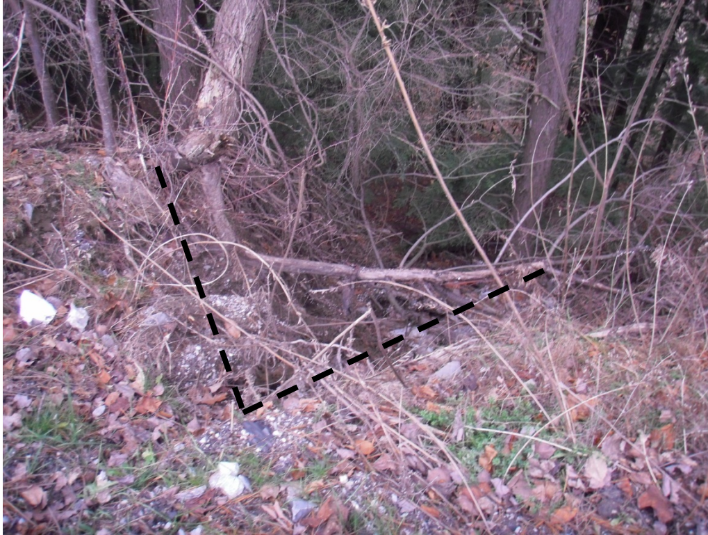
Figure 13. Erosion gully forming near repaired landslide at Highgate town sand shed.
